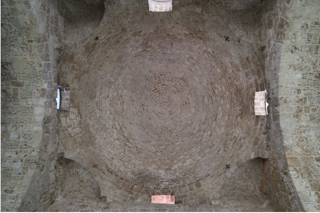
Fig. 1 - The dome seen from inside and from below (photo by Unicity S.p.A).
