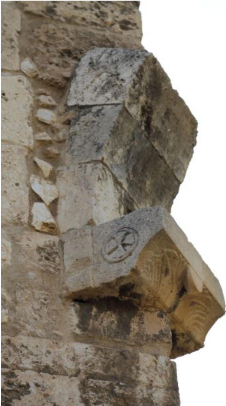
Fig. 1 - The broken shelf outside the domed structure (photo by Unicity S.p.A.).
