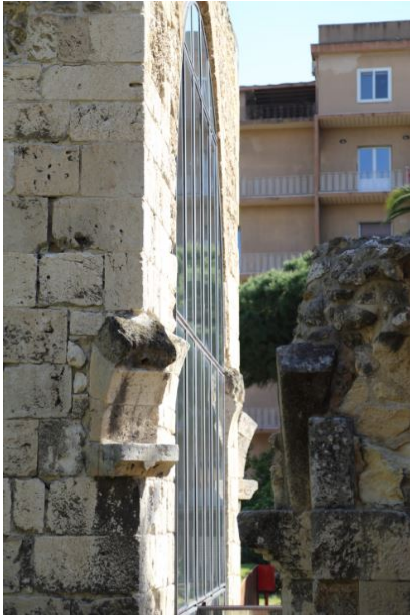
Fig. 3 - The shelves on the west side of the domed structure (photo by Unicity S.p.A.).
