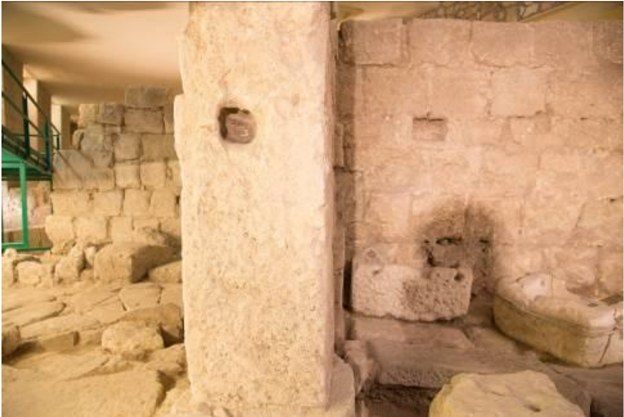
Fig. 3 - Jamb with hole for connecting element of the door in the home to the S-E (photo by Unicity S.p.A.).
