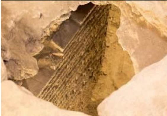
Fig. 2 - Inner sewer wall (photo by Unicity S.p.A.)
