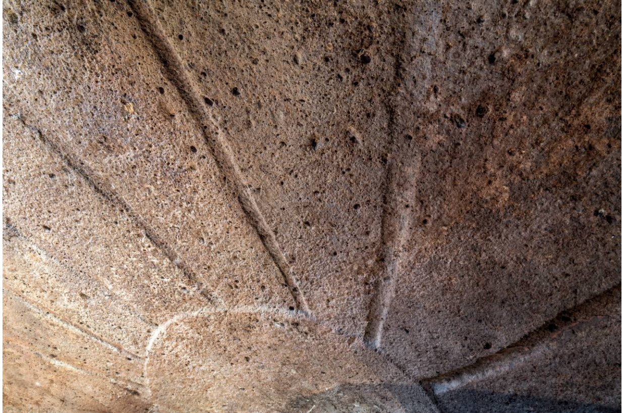
Fig. 2 - The ceiling of the ante-cell (photo Unicity S.p.A.).
