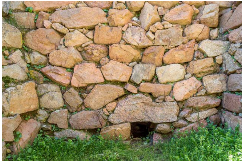
Fig. 3 - The canal in room B of the megaron 1 temple (photo by Unicity S.p.A.).
