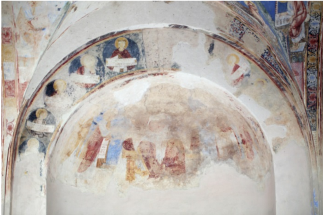
Fig. 2 - Frescoes in the apsidal vault: Christ in majesty (photo by Unicity S.p.A.)
