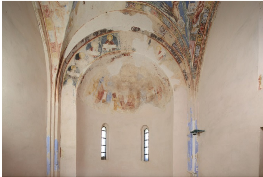
Fig. 2 - The apse of the church of San Nicola di Trullas (photo by Unicity S.p.A.).
