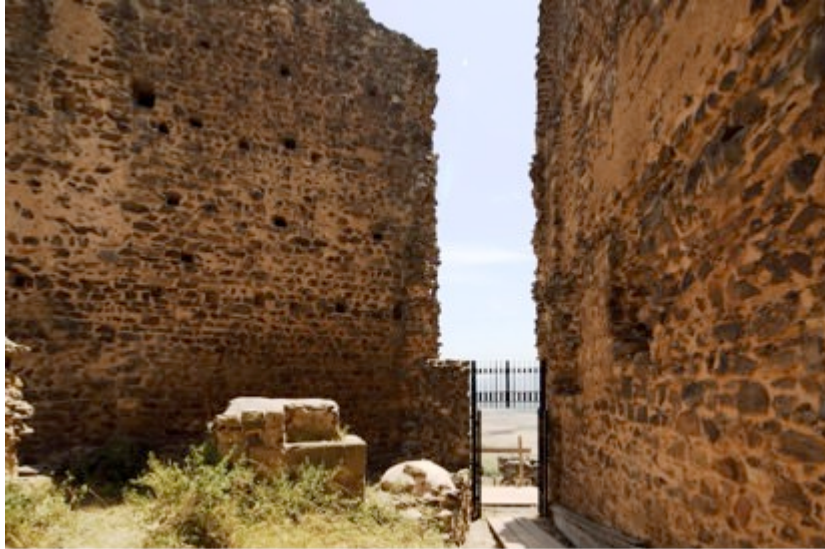
Fig. 9 - The entrance to the keep seen from inside after restoration (photo by Unicity S.p.A.).
