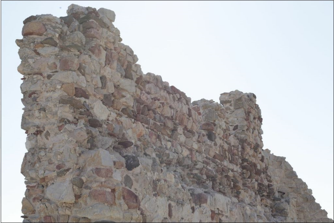
Fig. 2 - Detail of the walkway around the inner perimeter wall (photo by Unicity S.p.A.).
