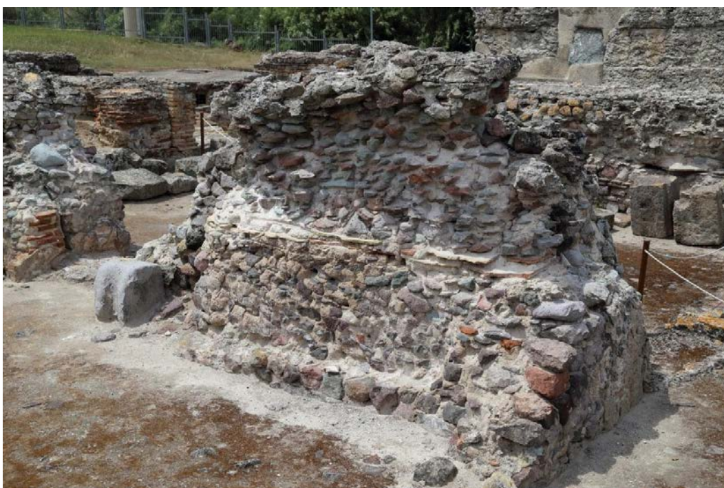
Fig. 4 - Wall of the tepidarium with evident signs of the bad erosion that has bared the wall's inner structure (photo by Unicity S.p.A.).
